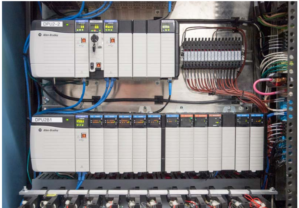
Figure 3. Time management. Upfront planning can reveal many ways to minimize downtime when migrating from an old DCS to a new automation system. This new system allowed existing field terminations to remain intact.
