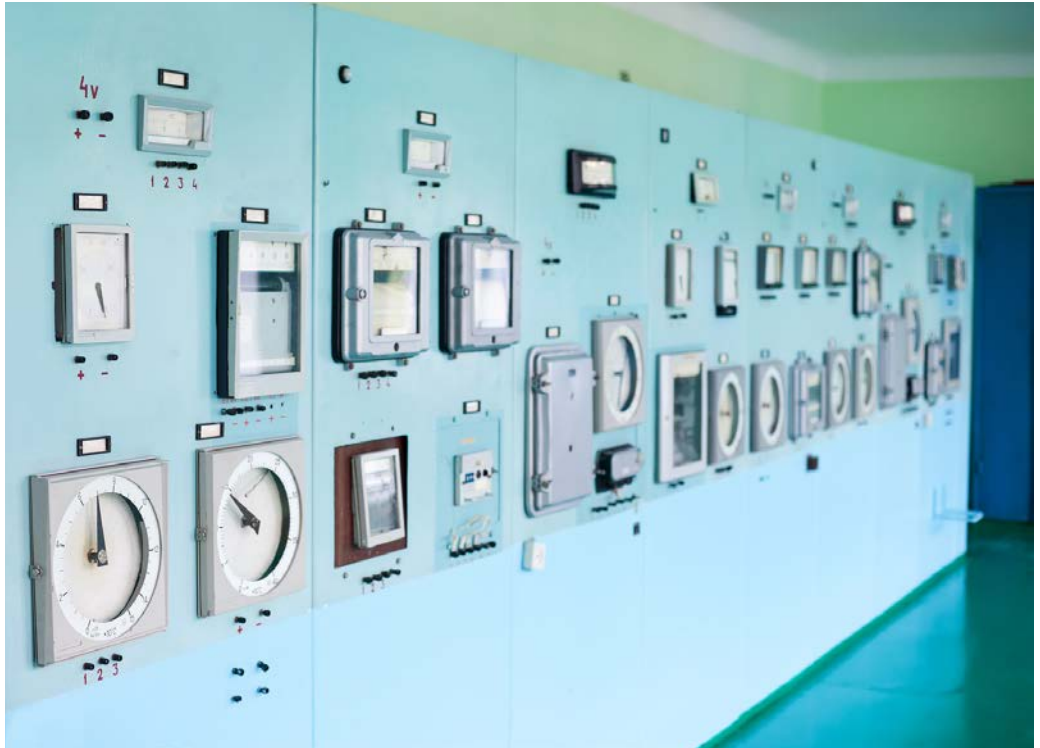
Figure 4. Old school. When operator interface panel boards are replaced with modern PC-based HMIs, extensive training is needed to bring plant personnel up to speed.
