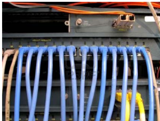
Figure 3. Major automation suppliers provide best practice information so the user starts with a sound network design for their control system.
